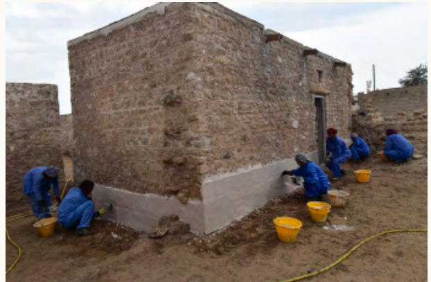
Figure 2: Restoration works on a traditional coral stone house in Al Jazeera Al Hamra
